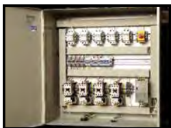
Electrical Safety Enclosure located at rear of System
